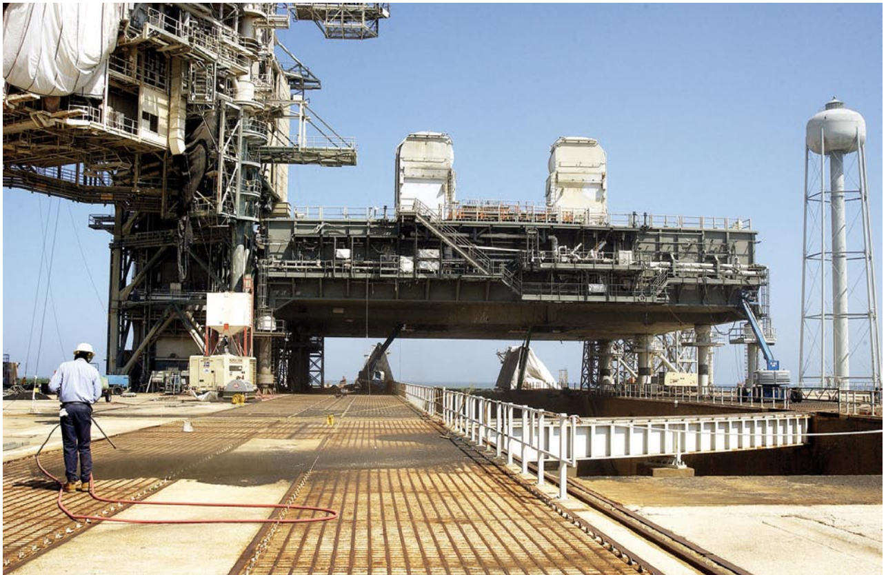
A worker sandblasts the surface behind the Mobile Launcher Platform on Launch Pad 39A . Routine maintenance includes sandblasting and repainting to minimize corrosion.
